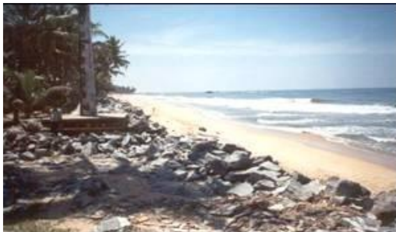
Photo 5.5 Stones Dumped as Temporary Measure
