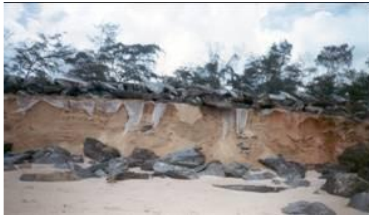
Photo 5.1 Inadequate Filter Layer
