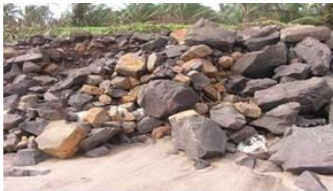
Photo 5.2 Pockets in Armour Layer
