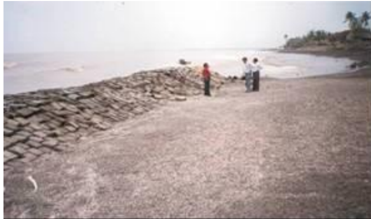
Photo 5.3 Pockets in Armour Layer
